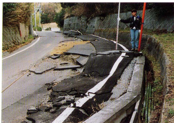
写真5. 地点⑪. 桃林寺下のアスファルト道路の破壊状況 Photo. 5 Destruction of paved road near Torinji Temple at Loc ⑪, Ezaki Village
