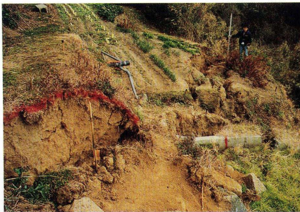
Photo. 32 Collapse of footpath at Loc ④⑥
