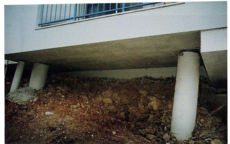
写真58. 地点⑧⑤. RC 建築の基礎杭のずれ Photo. 58 Deformation of supports of RC building at Loc ⑧⑤
