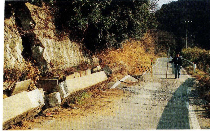
写真40. 地点⑥0. 県道の右 ずれ変位と側壁の破壊 状況 Photo. 40 Right lateral offset of road and de- struction of concrete wall at Loc ⑥0
