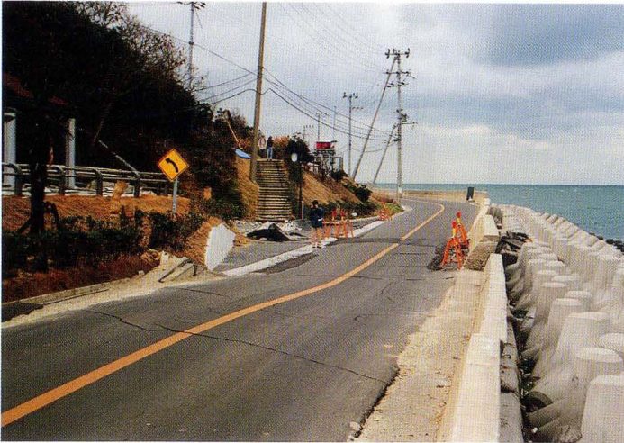
写真1. 地点①. 江崎灯台下, 県道の水平ずれと段差 Photo. 1 Lateral offset and throw of paved road at Loc ①, near Ezaki lighthouse
